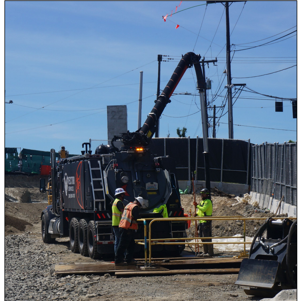
Workers using a vacuum truck to prepare the site for lid foundation construction north of SR 520 (June 2026)
