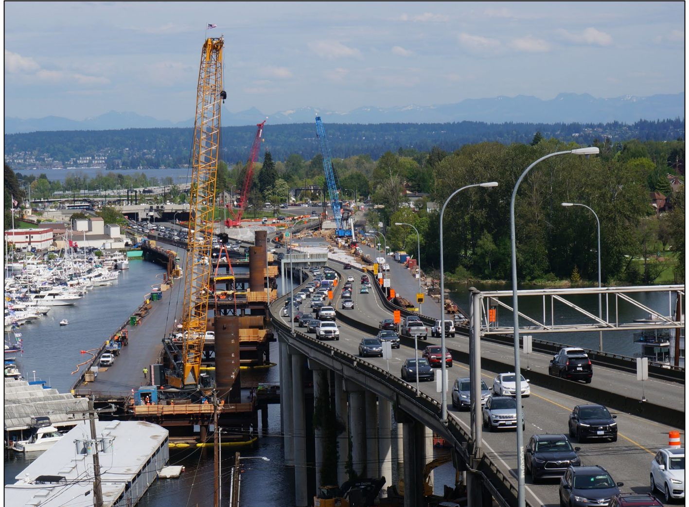
Crews install drilled shaft casings north of the Portage Bay Bridge (May 2026)
