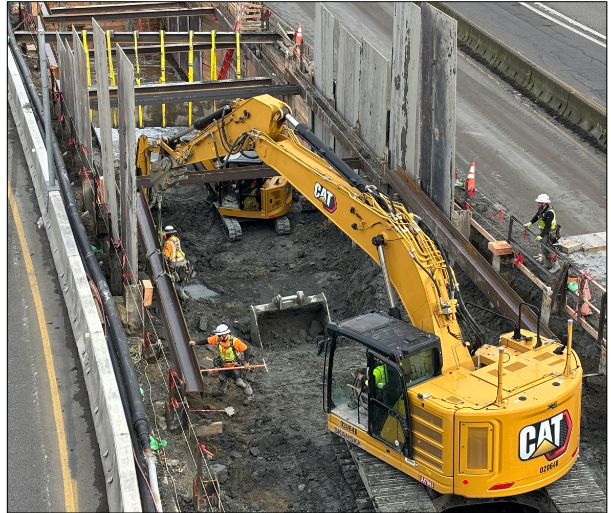
Crews excavating for the lid foundation between the east and westbound lanes of SR 520 (Jan. 2026)
