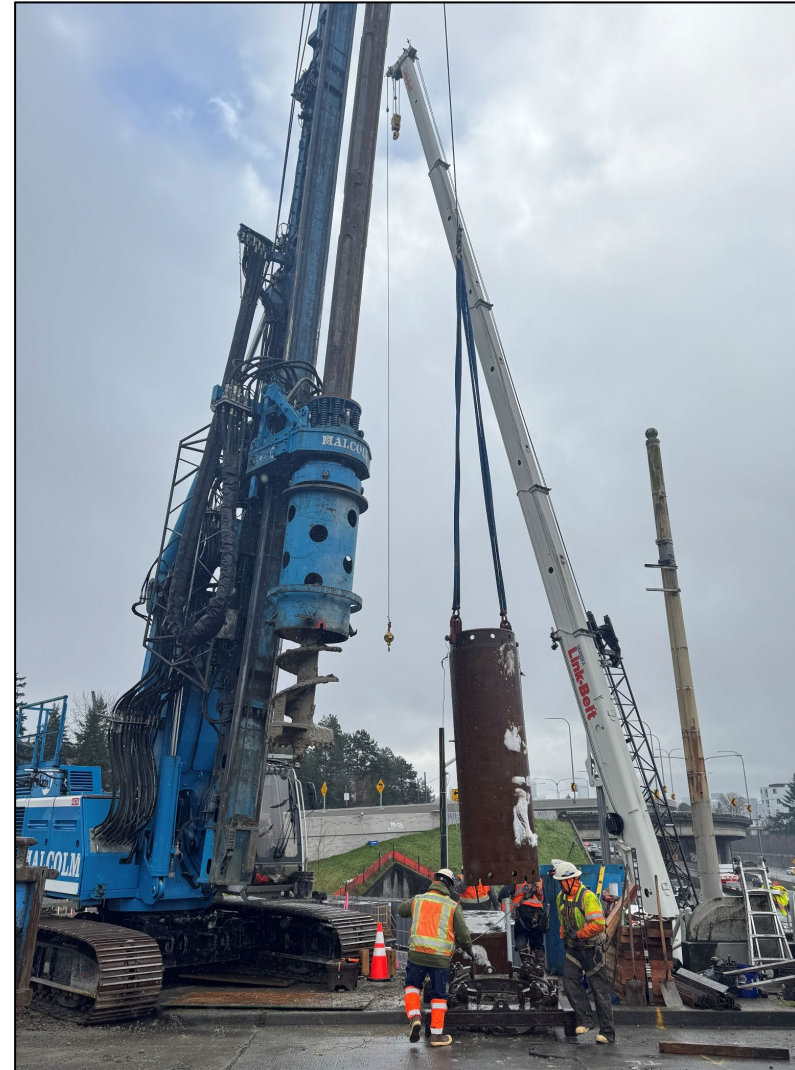
An example of the drilling equipment crews will use to construct the lid foundation (March 2025)
