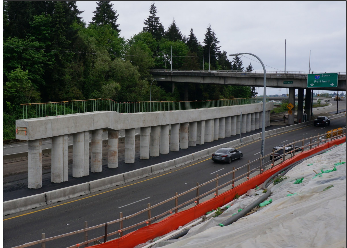
The completed section of foundation sits between 10th Avenue East and Delmar Drive East, between the eastbound and westbound lanes of SR 520 (May 2026)
