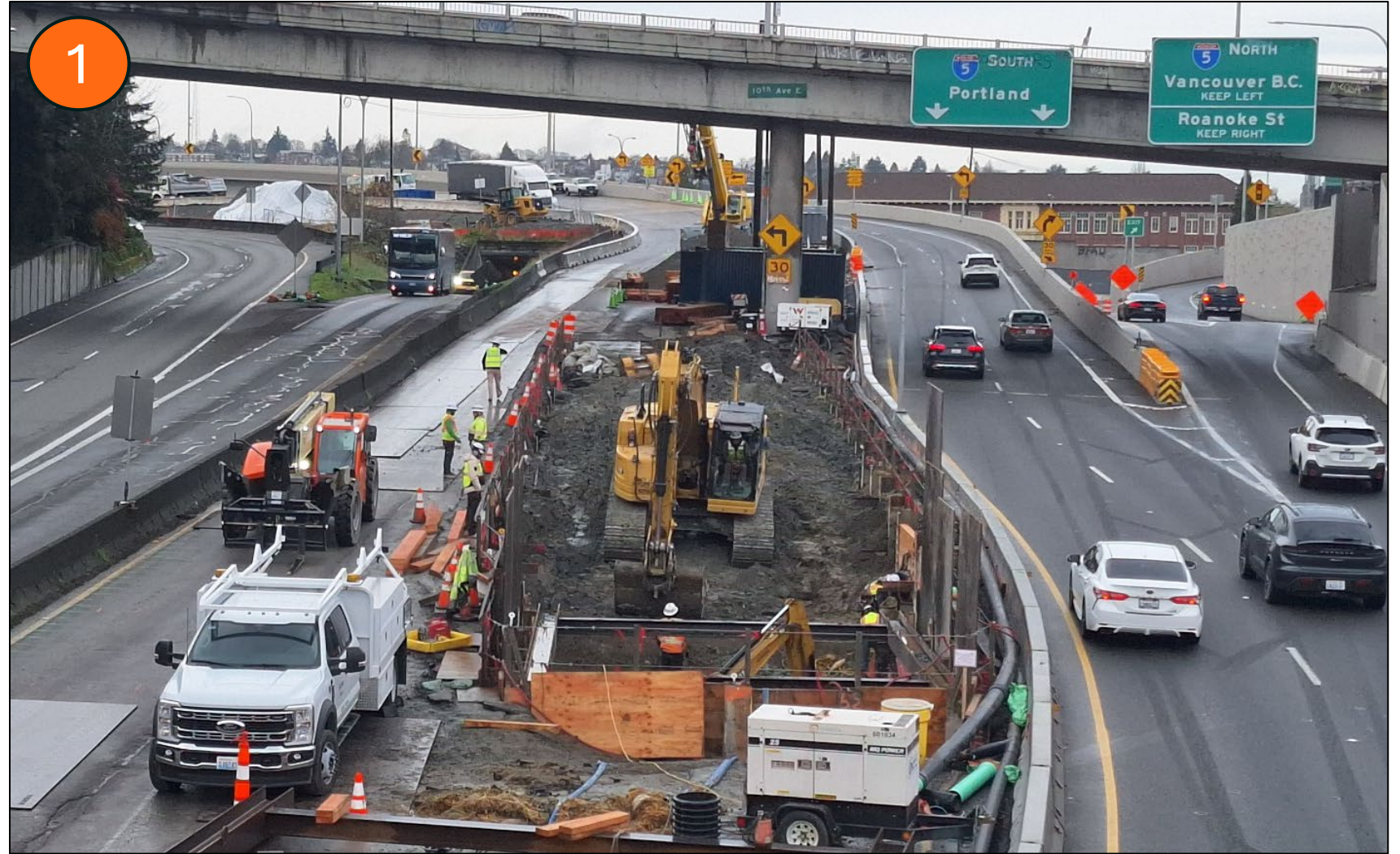
Crews excavating for the lid foundation between the eastbound and westbound lanes of SR 520 (Dec. 2025)
